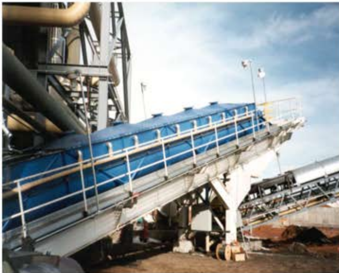
Self-contained "HOLO-SCRU" Coolers handling Fly Ash with water spray capabilities
